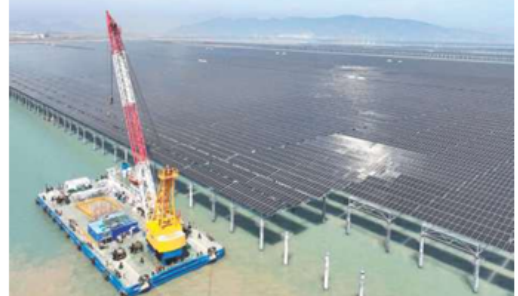
Towards sustainability: Solar panels being placed at the CNNC Tianwan tidal flat photovoltaic power plant in Lianyungang, in China's eastern Jiangsu province, on April 19.
