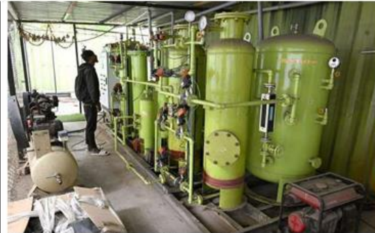
A biogas plant at the Waste-to-Energy unit in Koramangala in Bengaluru. J. ALLEN EGENUSE
